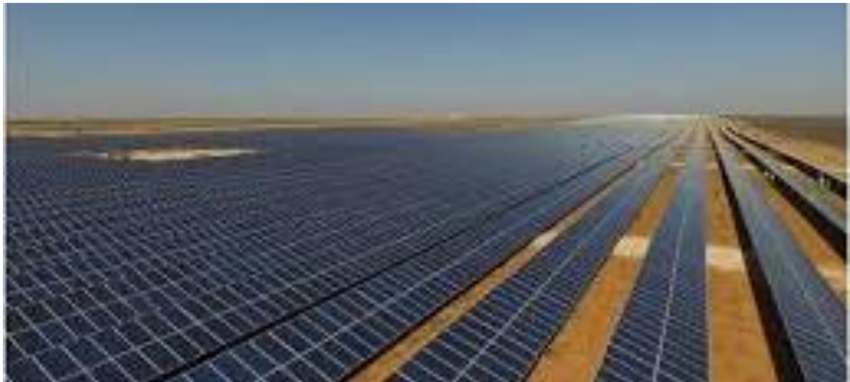
NP Kunta Ultra Mega Solar Park (978.5 MW)
