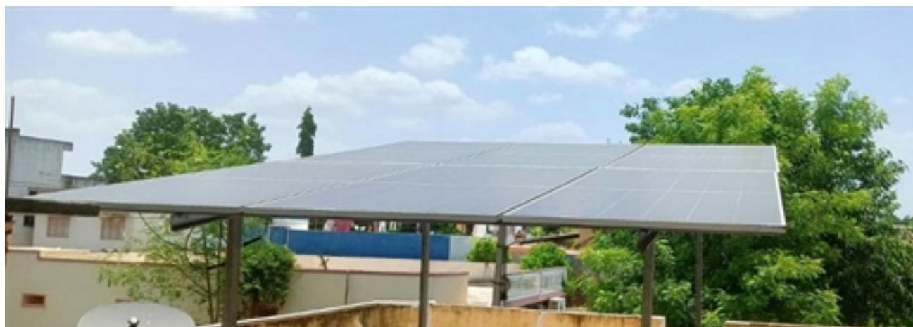
Solar Rooftop Unit
