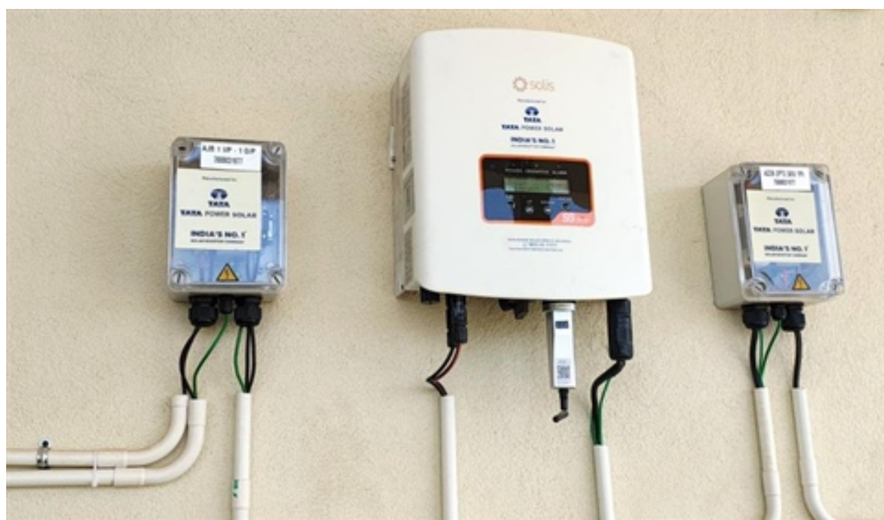
Solar Rooftop Net Metering
